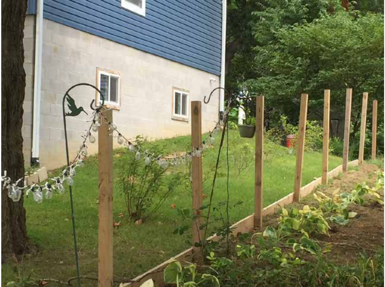
Shows level of where top of fence would be. These posts were put in by Fikes as part of Drainage wall. They are right on the property line. The distance between the houses is approx. 20 feet.
